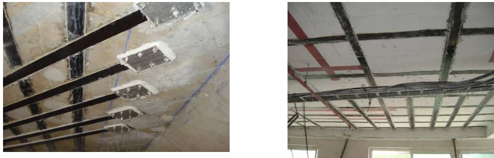
Fig 5 Use of Laminates in for strengthening of slabs in a bridge and a building.
